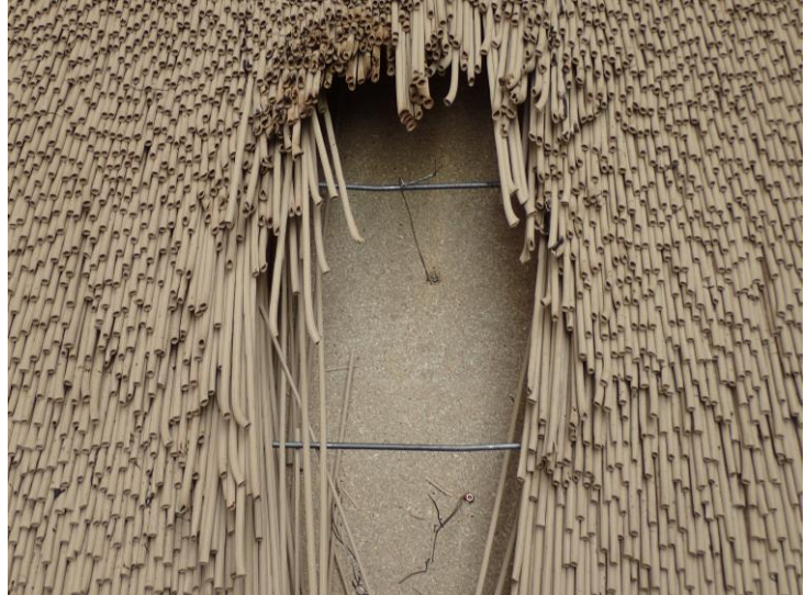
Photo 12 The undamaged section of the supporting deck of test specimen 3.
