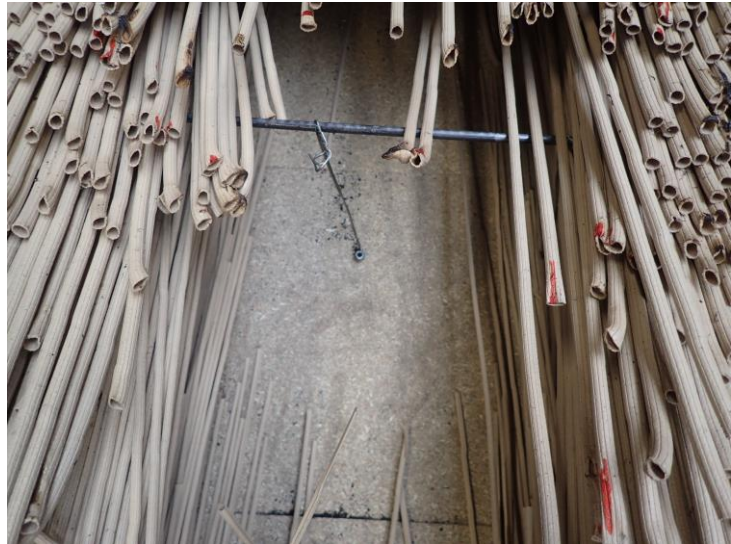
Photo 10 The undamaged section of the supporting deck of test specimen 2.
