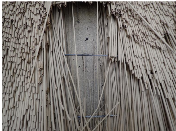
Photo 8 The undamaged section of the supporting deck of test specimen 1.
